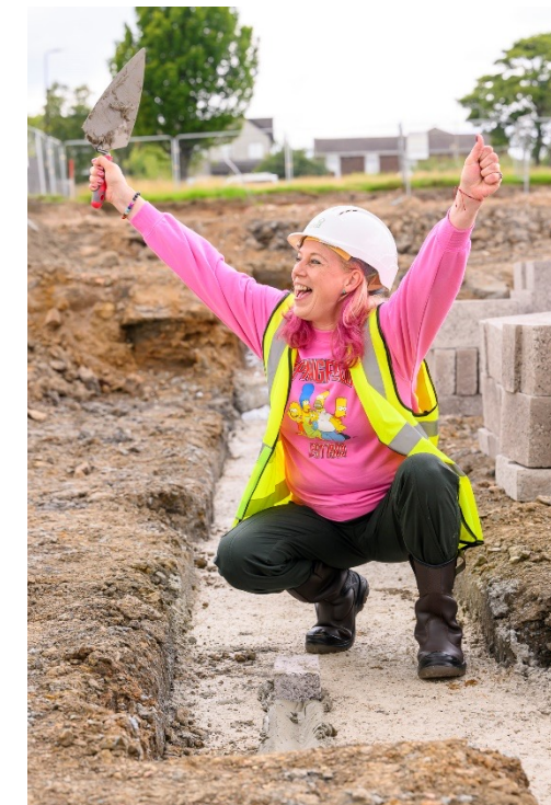
Springfield Properties - Deans South resident places first brick of her new home
